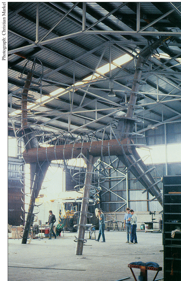
Deborah Halpern, Angel under construction at Shed 14, Victoria Dock, Melbourne, showing steel armature 2 prior to cement skin and application of tiles, 1987
